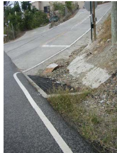
Figure 6 – Accumulated Debris Upstream of Outfall to Coral Harbor
