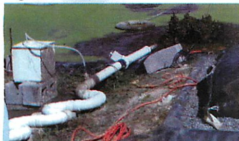
Figure 4. Effluent being pumped from the storage pond and injected with polymer prior to entering the geotextile bag. The white box houses the peristaltic pump which injects the polymer. The effluent coagulates as it mixes with the polymer in the series of 90-degree PVC elbows.
