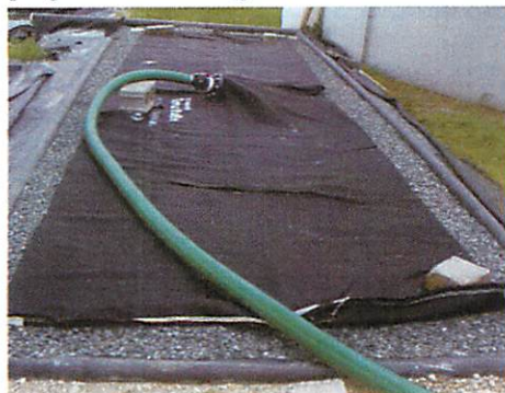
Figure 2. The geotextile bag resting on the earthen pad. The green, 3-inch PVC hose delivers effluent injected with polymer to the bag.
