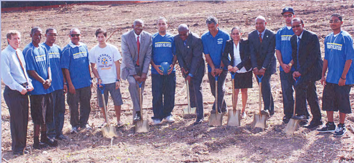
Members of the UVI Soccer Team, UVI administrators and government officials "break ground" for the Albert A. Sheen Campus' soccer fields on St. Croix.
